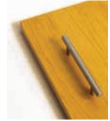
Step 5 The jig is now set up for all doors in the kitchen and each door can quickly be marked out ready for drilling
