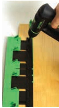
Step 3 Using either a 2 mm pilot drill bit or an awl, mark the door where the first hole is required
